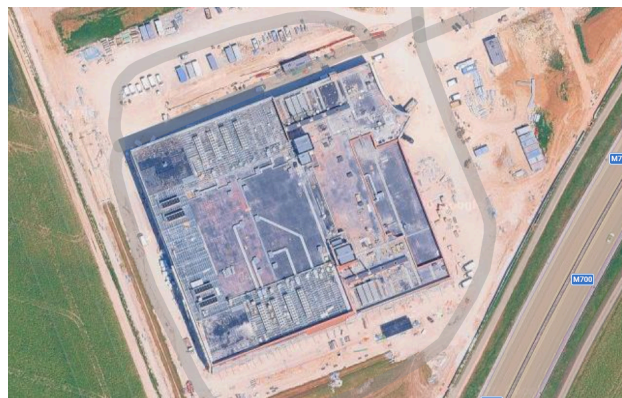
Satellite view (Google Maps) of the Credit Mutuel data center construction site in Fauverney
